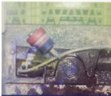
CRATE-WASHING CONVEYOR IN DAIRY
